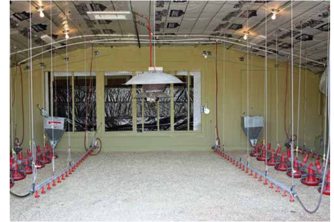
(top) MSU Student Broiler Barn for training future live production service techs (provided by BankPlus).
